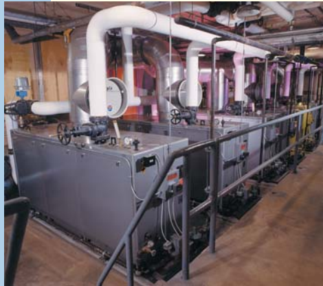
Six Bryan Boilers replace two 300 HP boilers at Carver Senior High School, New Orleans, with six stage lead-lag system matching output to demand, for maximum economy.
