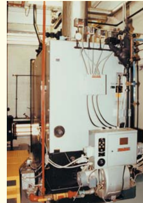
At a major office furnishings manufacturer, this Bryan Boiler provides clean, dry, steam to process toxic solvent bearing chemicals for safe disposal.
