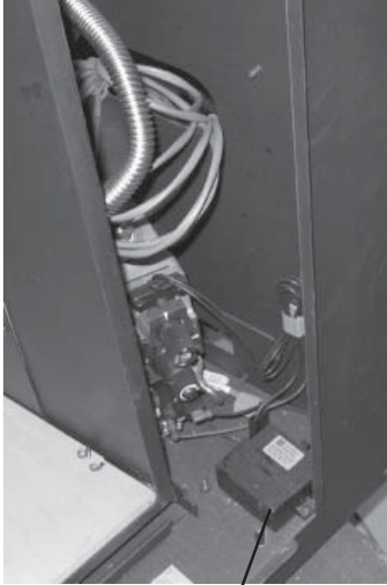
DC Spark Box Location
